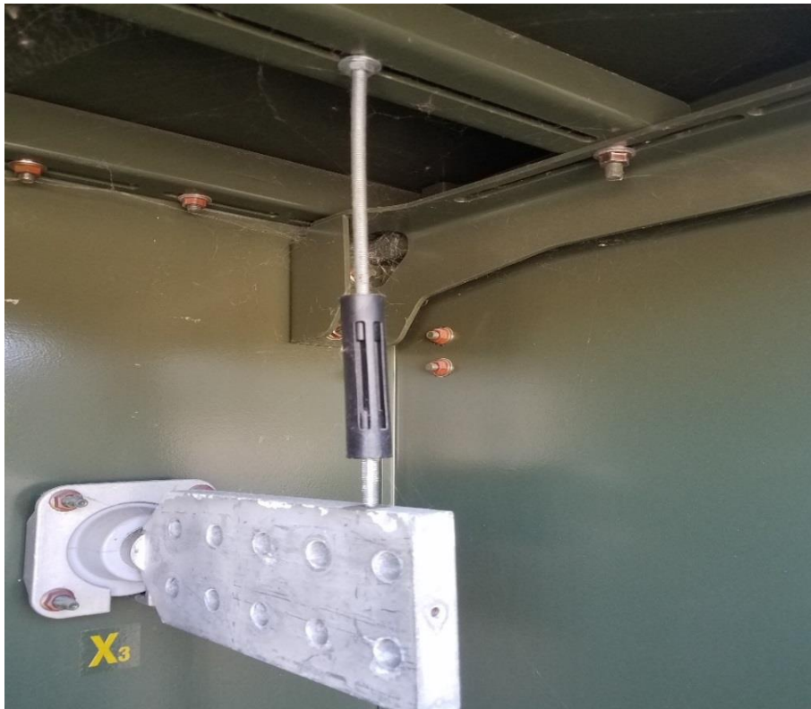
Figure 4 - Insulated paddle support for transformer secondary
