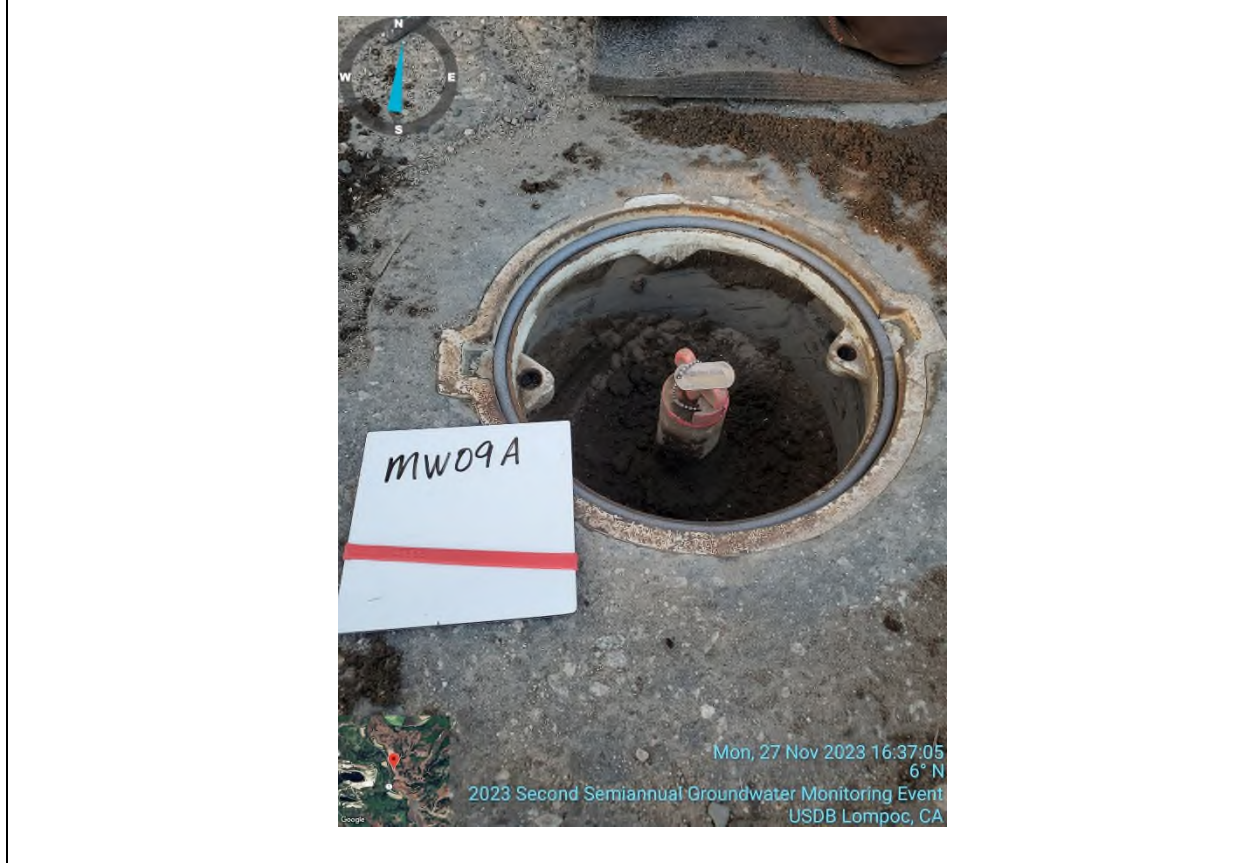
Photo #6: Condition of WR-MW-09A after well maintenance. Gasket replaced and dirt removed from well box.
