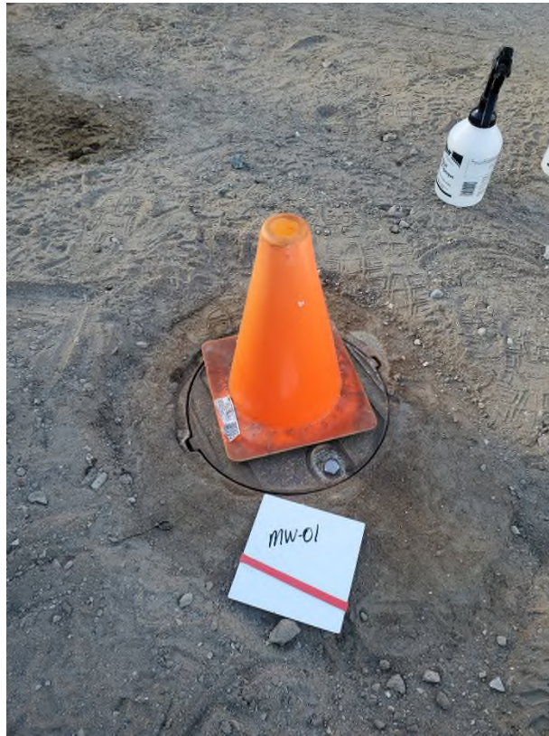
Photo #11: Condition of WR-MW-01 after well maintenance. Repairs were attempted on the well lid tabs but unable to re-thread sufficiently.
