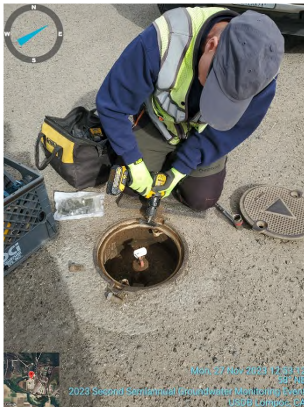
Photo #4: Performing maintenance on well box — Removing dirt buildup using a steel-head rotary brush.
