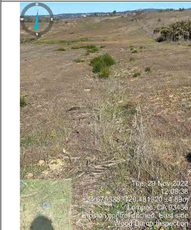
Photo 9: Eastern Erosion Control Lined Ditch - smooth grade and minimal obstructing vegetation (facing north)
