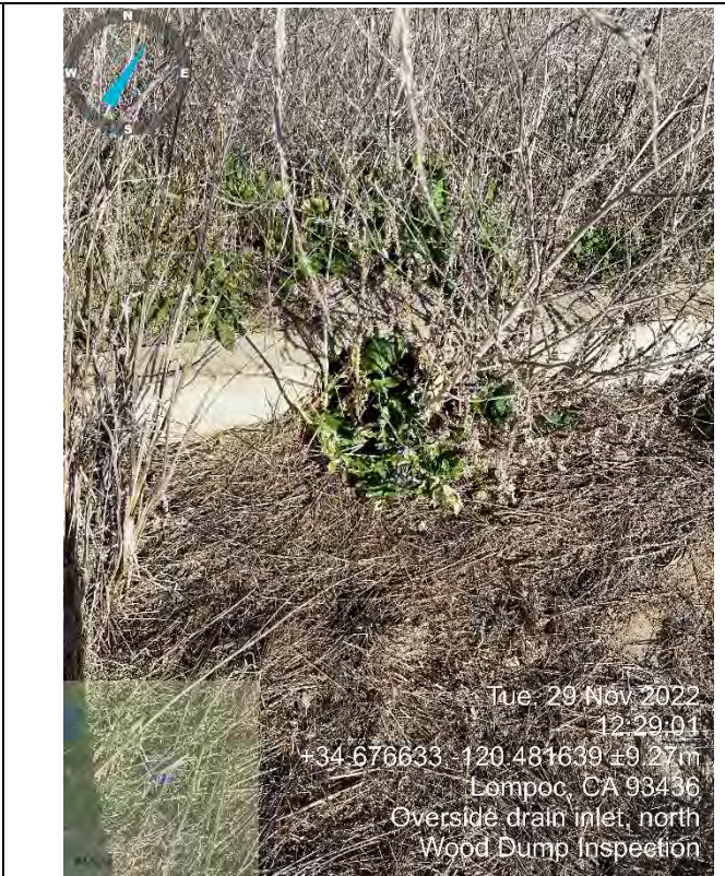
Photo 16: Northern Overside Drain Inlet obstructed by vegetation (facing northeast)
