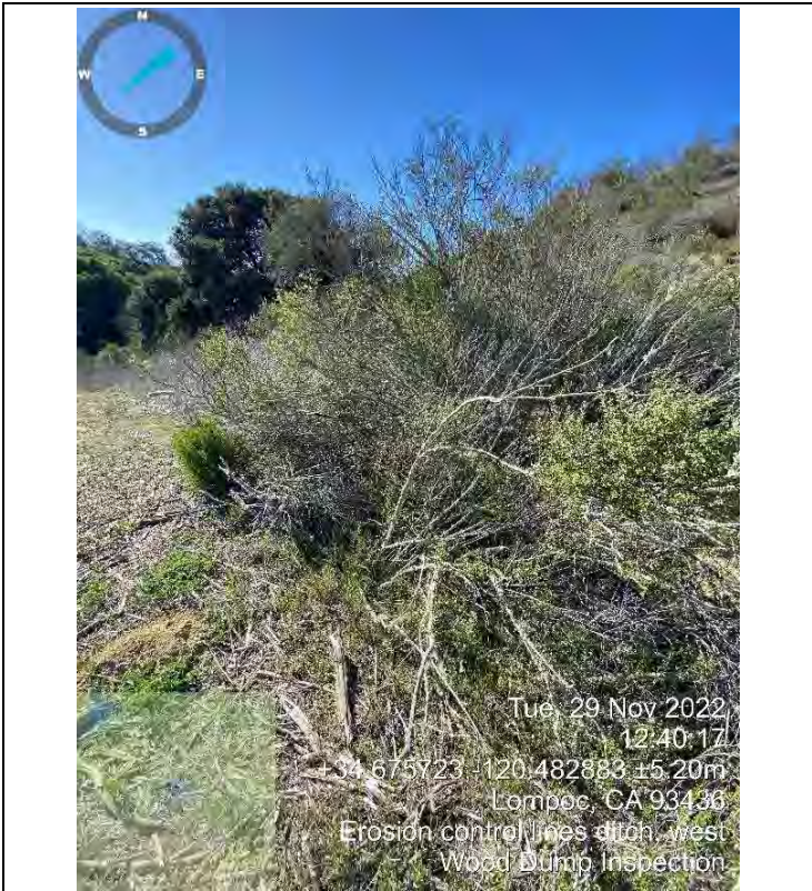
Photo 19: Western Erosion Control Lined Ditch – woody vegetation obstructing ditch at southern end (facing southwest)
