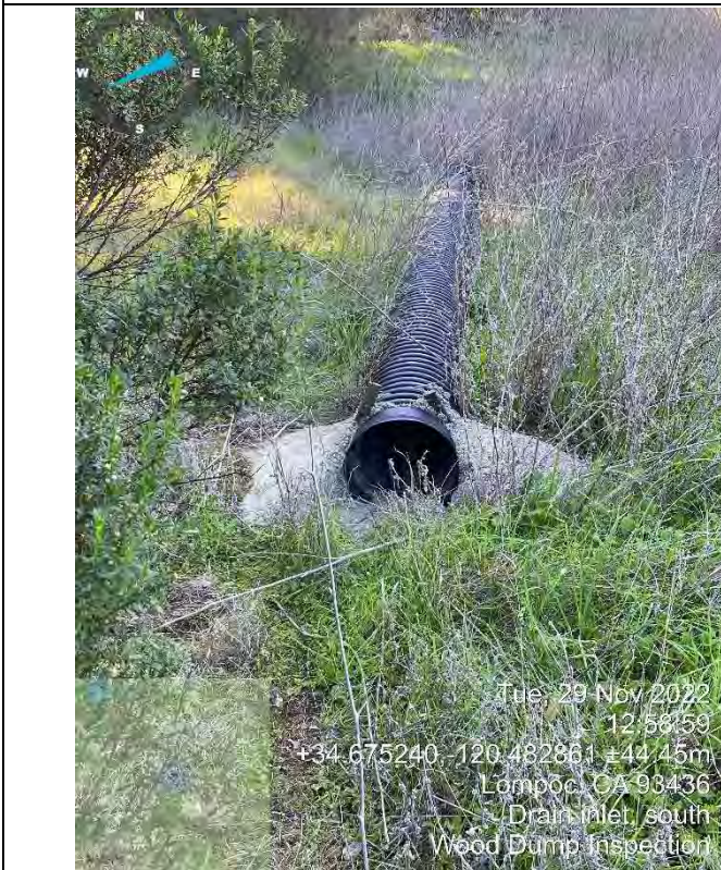
Photo 29: Southern 12" HDPE Pipe Inlet– pipe in good condition, well anchored, and unobstructed (facing southwest)
