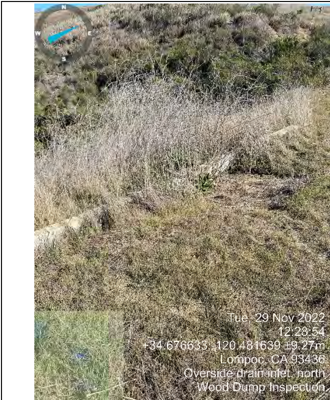
Photo 15: Northern Overside Drain Inlet and Wingwall – concrete in good condition (facing northeast)
