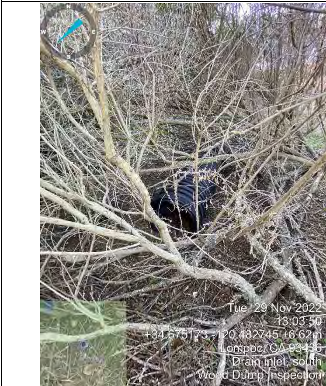
Photo 33: Southern 12" HDPE Pipe Inlet - pipe in good condition but obstructed with vegetation and debris buildup (facing southwest)
