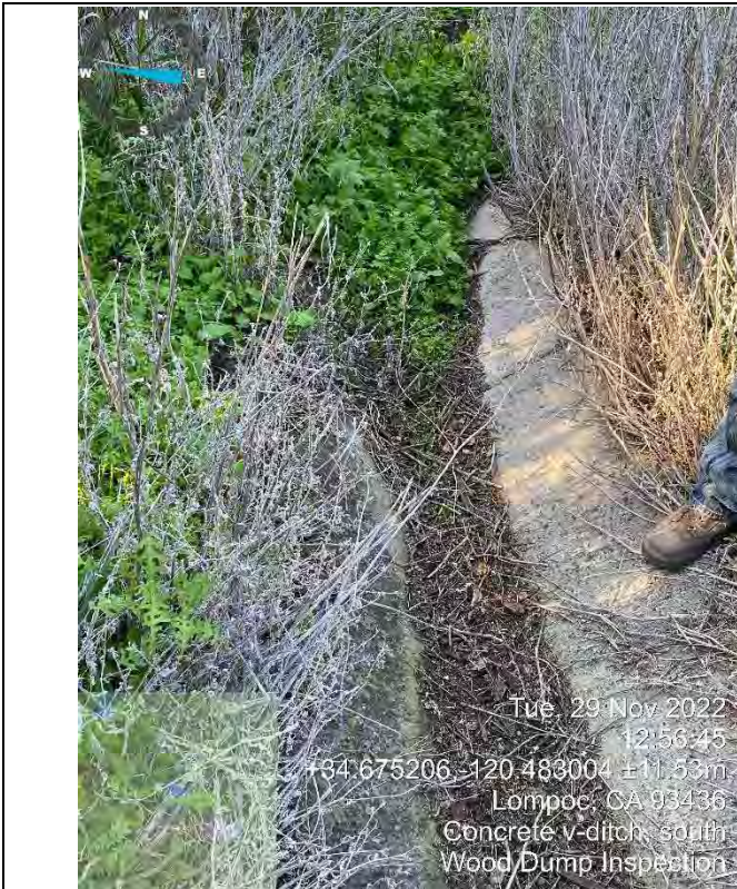
Photo 27: Southern Concrete V-Ditch – concrete is undamaged but obstructed by soil and vegetation buildup (facing west)
