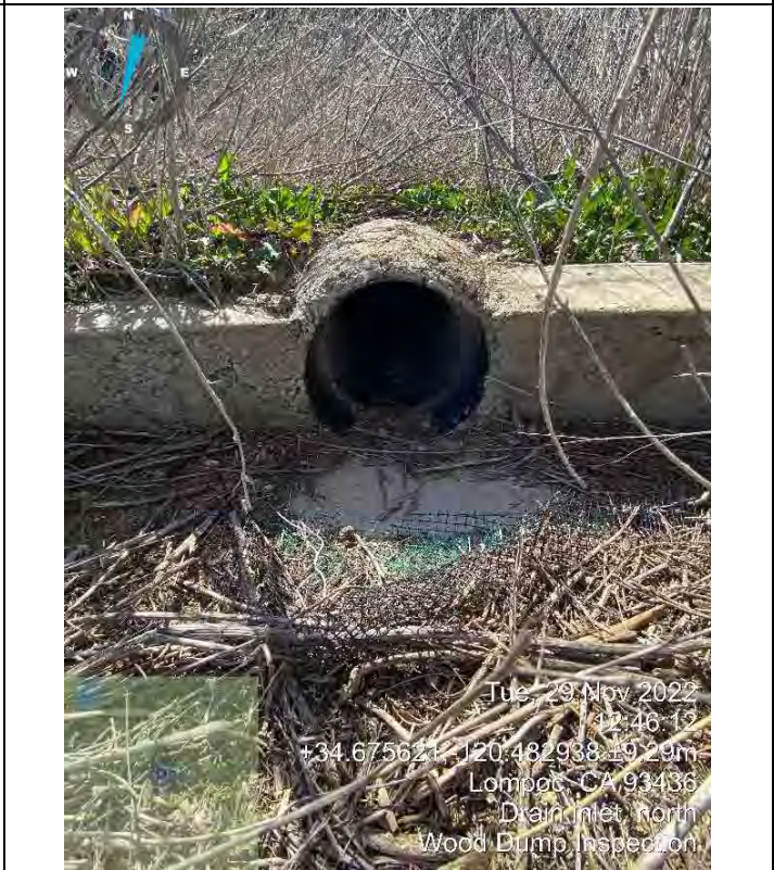
Photo 22: Southwestern Overside Drain Inlet – pipe is in good condition with no signs of obstruction at the opening (facing south-southwest)
