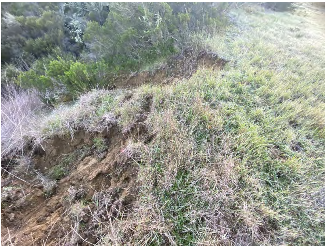
Photo 2: Close-up view of erosion on slope at the Wood Dump Area. January 2023
