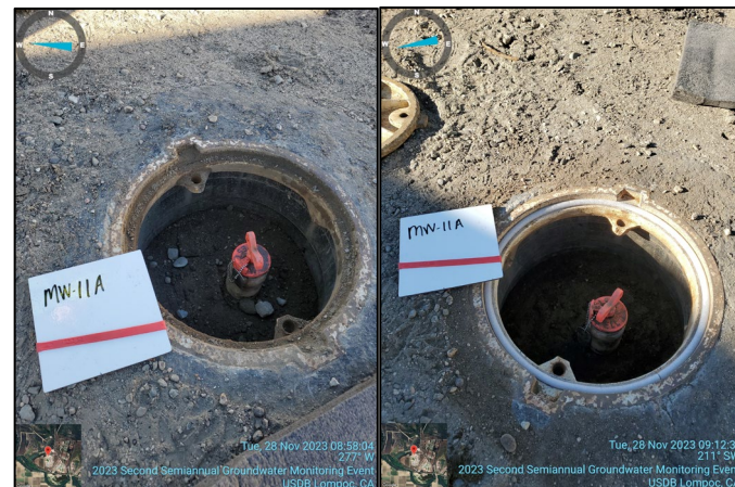
Before and after well maintenance performed to prevent soil and water infiltration into well boxes. Included new gasket, re-taped threads, and new bolts
