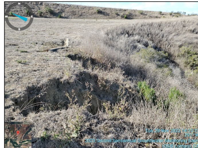
Erosion at northern drainage inlet in foreground, Wood Dump cover in background
