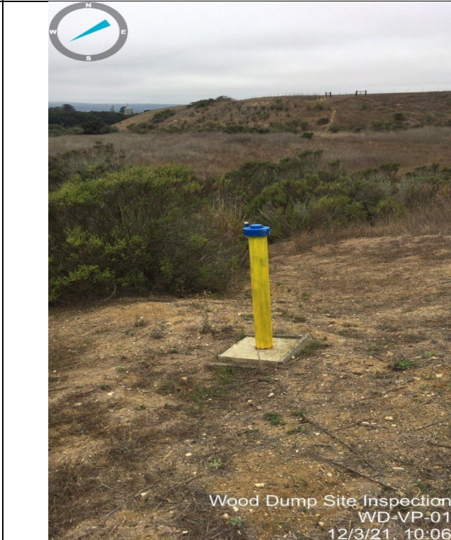
Photo 16: Vapor probe, WD-VP-01, facing southwest.
