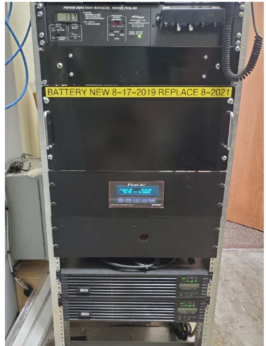
Notes: Tone Alert System- Westnet First-In Alert System: Master Control Unit: FIN-Eth-T10.
