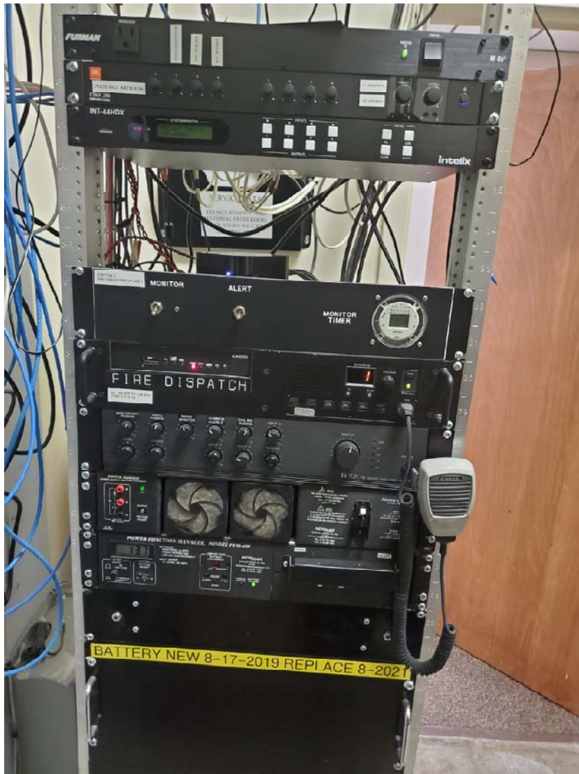
Notes: Radio: Kenwood TKR-750, Power Function Manager: Newmar PFM-400, UPS: Newmar 12-70. Backup Batteries 2-12VDC
