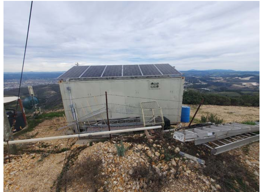
Notes: Ham radio equipment shelter and antennas.
