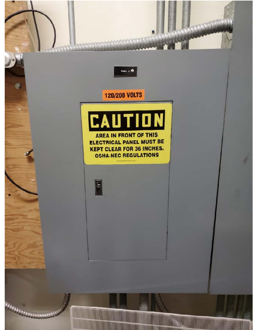
Notes: Outlet's Power Panel "E" Breaker 17 20amp breaker
