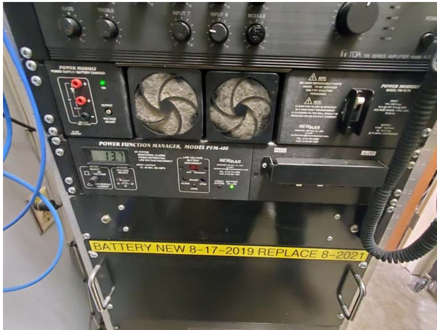
Notes: Power modules- PFM 400 and PM-12-70
