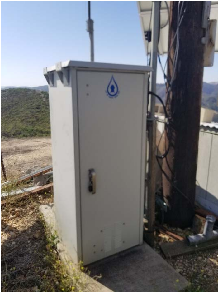
Notes: Housing Shelter for City LMR/SCADA equipment
