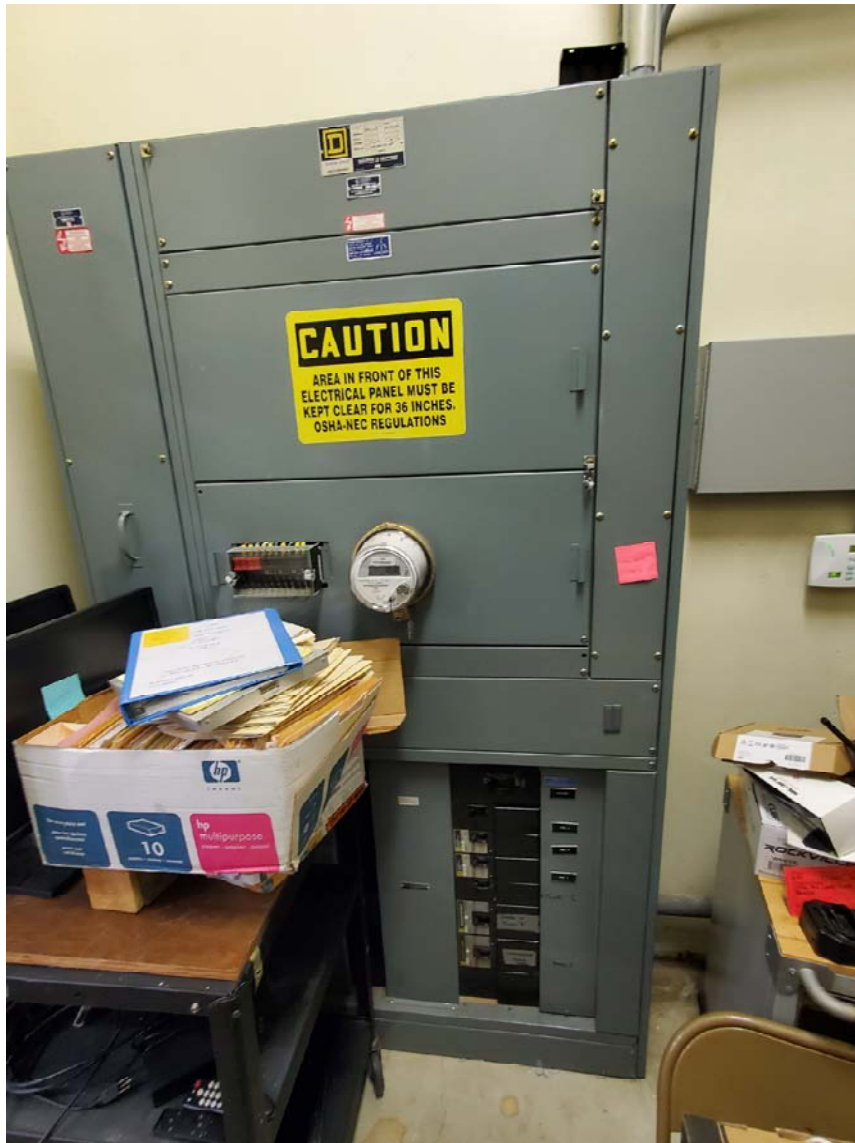
Notes: Main power panel to the build
