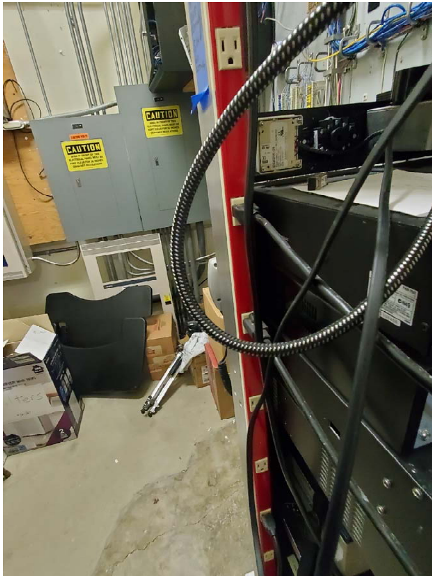
Notes: PFM is connected to 120VAC power strip.
