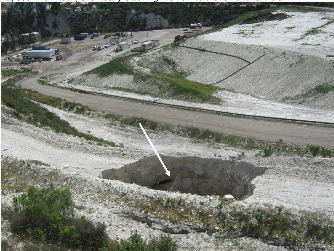
Photo 2 – Side view of eroded hole in drainage channel. Arrow points to an area that broke through and drained to lower drainage channels. Stormwater flowed to lower channels until the hole collapsed in on itself, eventually blocking the flow to the lower channels.
