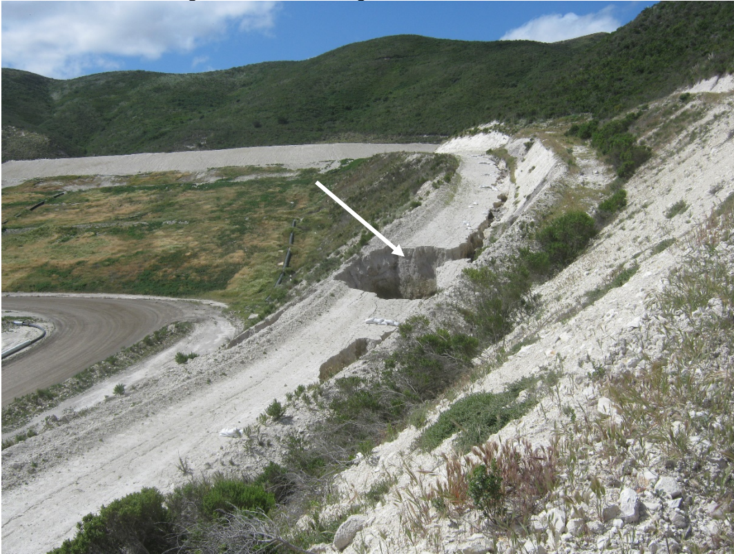
Photo 1 – West side drainage channel with large eroded hole.
