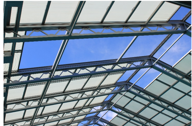
Competition Pool Ceiling Panels
