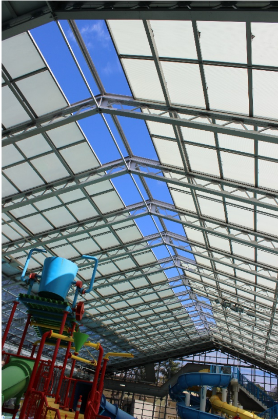
Activity Pool Ceiling Panels
