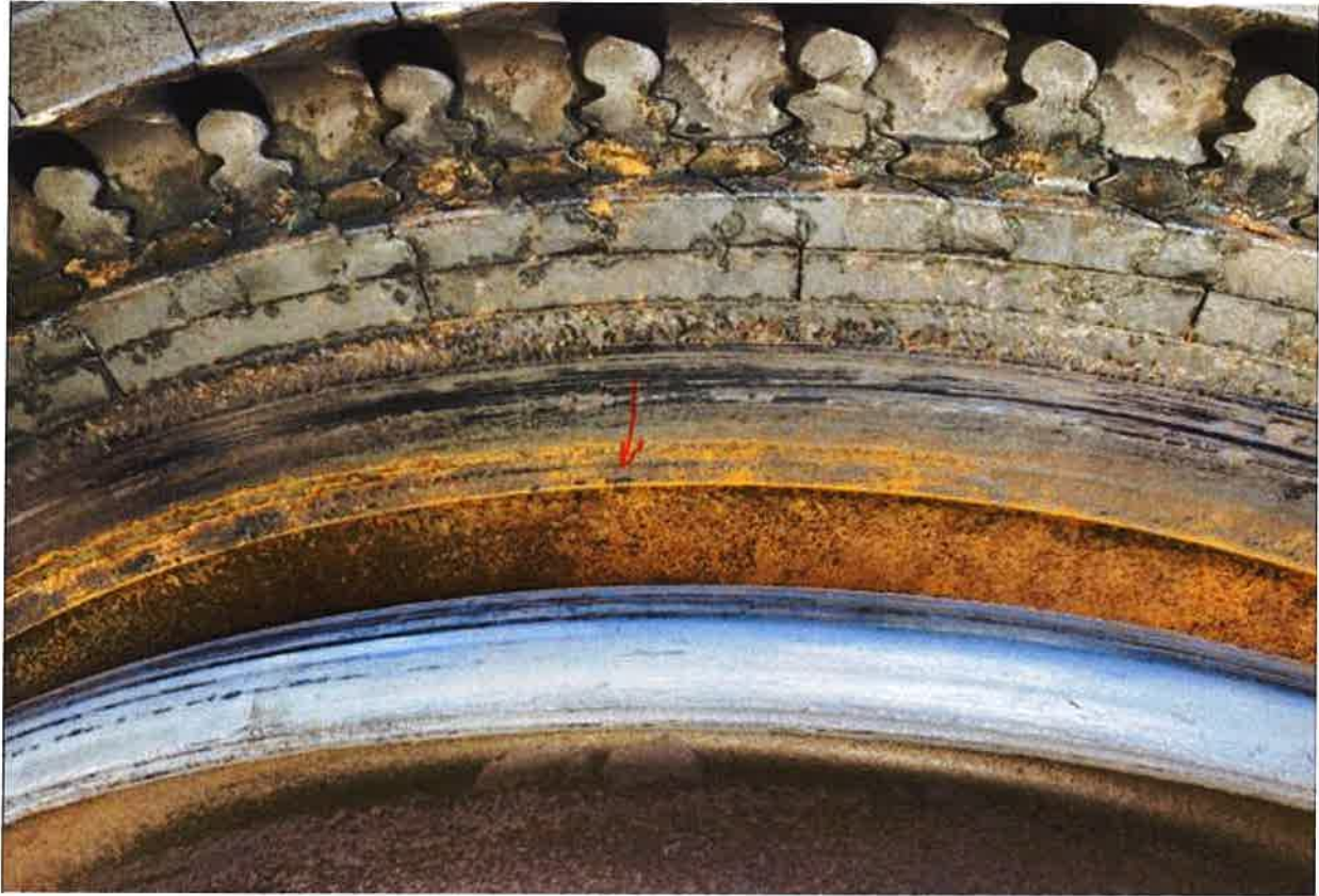
The Air Separator Housing melted in some locations.
