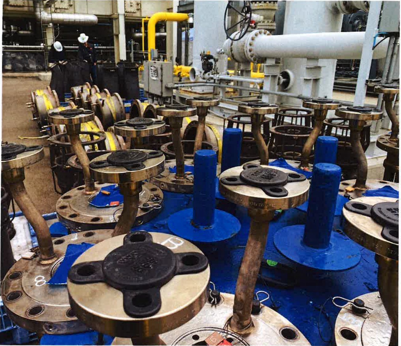
These are the rotor disks for the compressor section. The blue/purple colors are signs of heating. The arrows point to deep rubs with the seals.
