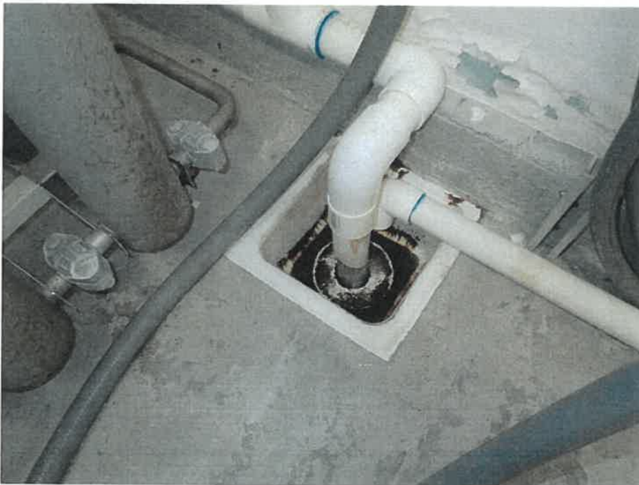
Photograph 2 – Drain Receiving Reverse Osmosis Reject and Spent Dialysate
