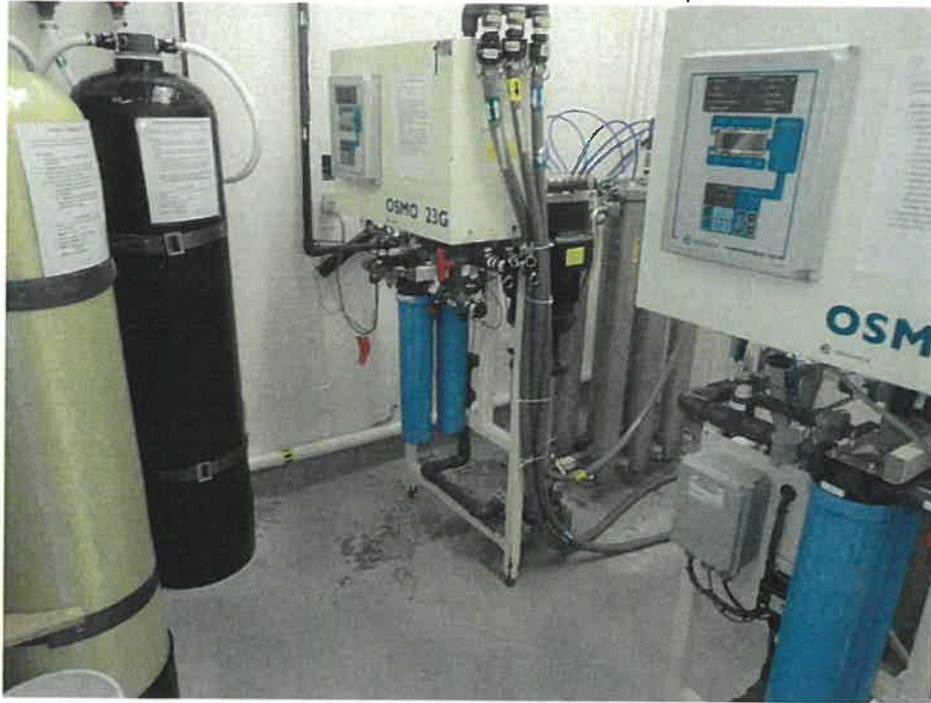
Photograph 1 – Water Treatment Equipment Labeled with Operating Instructions
