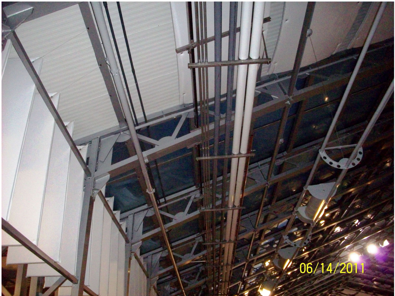
Pool Enclosure – Pipe Hangers with Conduit & Plumbing Piping
