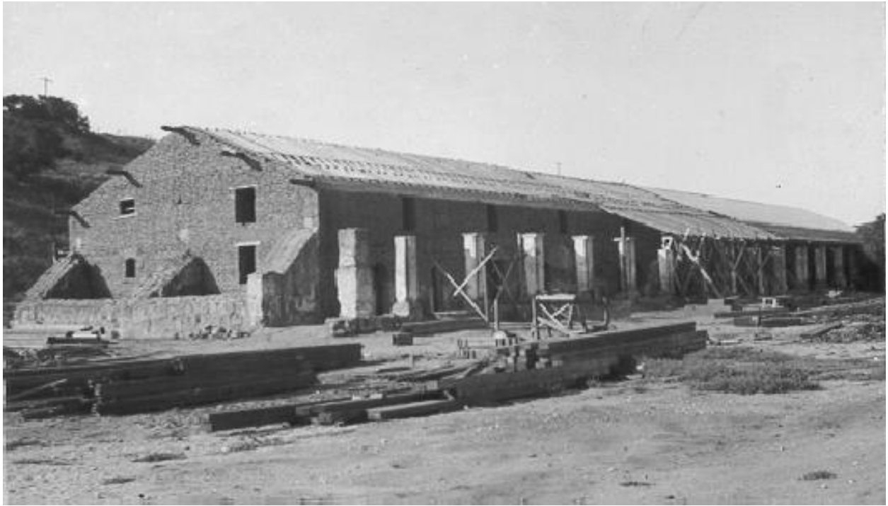
The reconstruction of the Mission residence building in 1935. This was the initial phase of the project.
