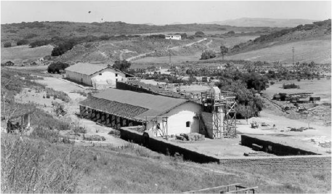
A photo dated 1938 of the later phases of reconstruction. Notice the scaffolding and the lack of roof on the center building.
