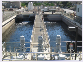
L1 - SEET/SEEPS: temporarily stores wastewater when the flow exceeds 5.5 MGD. When the flow falls below 5.5 MGD, the SEEPS pumps the wastewater to the filtration/ultraviolet (UV) disinfection systems.
