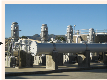
2 - IPS: Four variable speed nonclog mixed flow vertical column pumps are used to pump raw sewage into the Plant for treatment.
