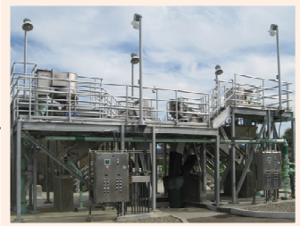
3 - Grit removal: flow from the IPS enters the grit removal system where heavier, inorganic material (grit) is removed before it enters the oxidation ditches. The grit is washed, dewatered, and disposed at the City's landfill.
