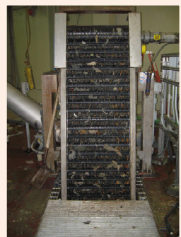
1 – Preliminary treatment: bar screens are used to remove large objects like sticks, rags, plastic, rocks, toys or trash to protect downstream processes.
