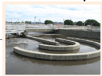
4 - Oxidation Ditches (OD): liquid waste stream from the grit removal system flows to the oxidation ditches where blowers provide air for the oxygen-breathing (aerobic) microorganisms start to break down organic matter and nutrients thereby removing pollution.
