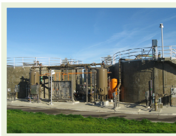
L1 - SEET/SEEPS: temporarily stores wastewater when the flow exceeds 5.5 MGD. When the flow falls below 5.5 MGD, the SEEPS pumps the wastewater to the filtration/ultraviolet (UV) disinfection systems.
