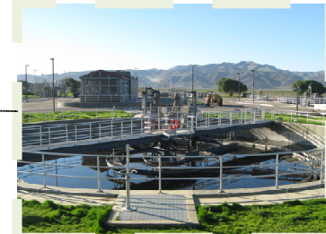
5 - Secondary clarifiers: the waste stream flows from the oxidation ditches and splits into three secondary clarifiers where heavier material (sludge) sinks and lighter material (scum) floats and is further treated. Settled sludge is returned to the OD.
